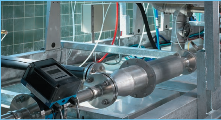
The water temperature can be controlled by a steam jet heater.
